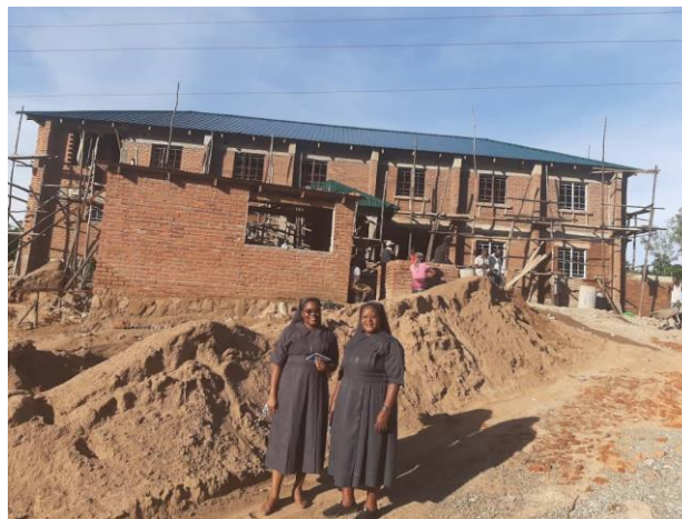
Teresian Sisters in front of their first hostel while it was under construction
